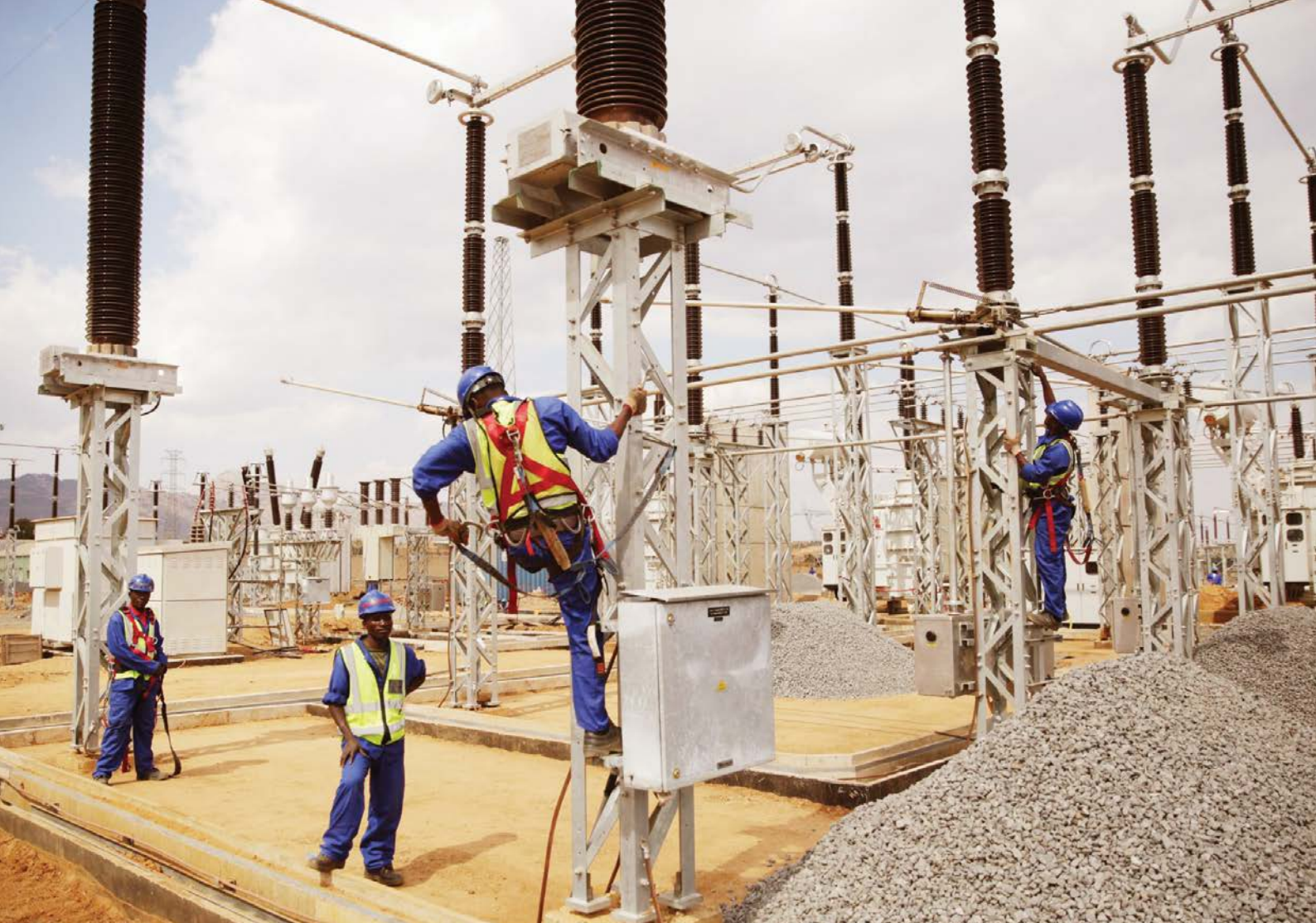
POWER: One of Malawi's electricity transmission stations
